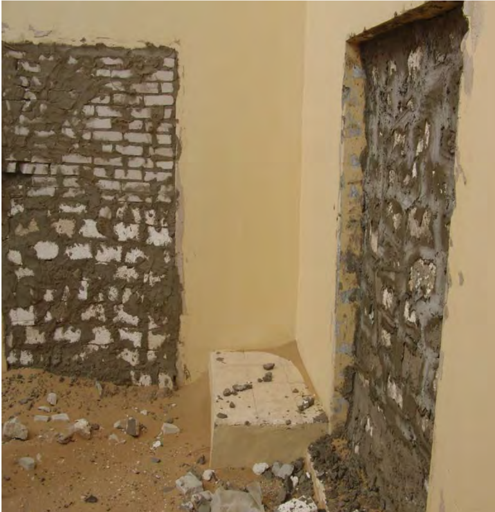
15. The damaged de Morgan storage facility Dashur with bricked doors. 15 February 2011. Photo Joris Kila.
