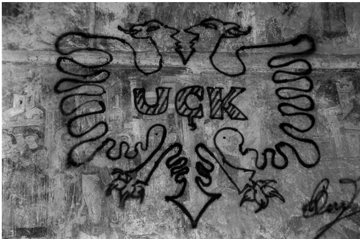
FIG 5.1 DAMAGED MURAL IN MATEJCE.
