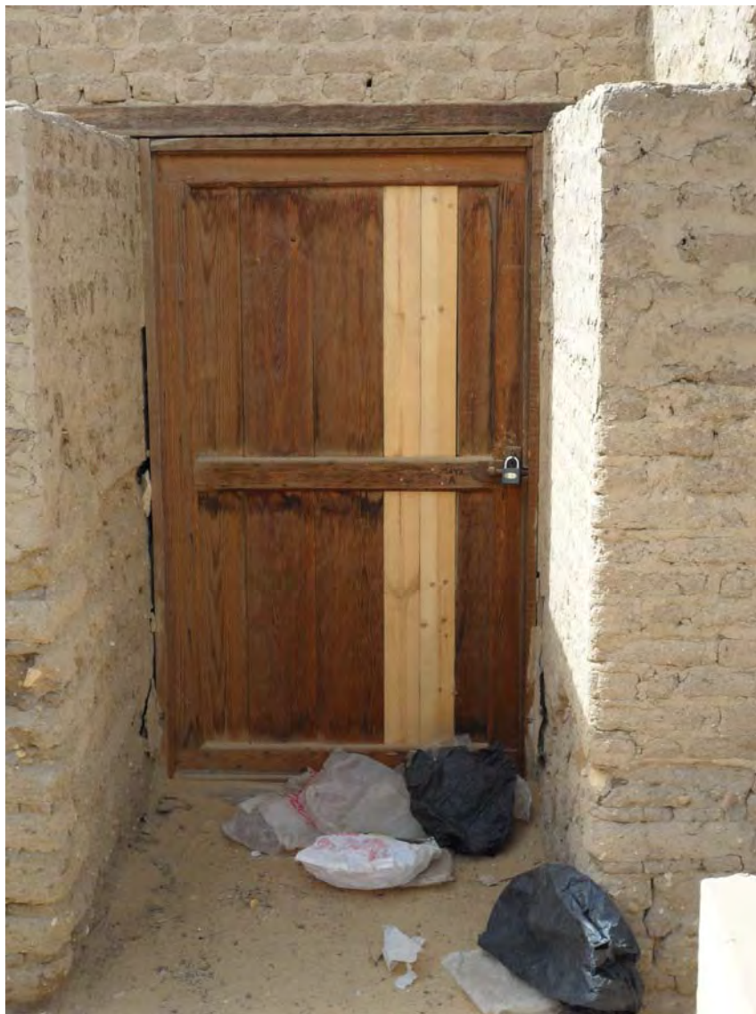
12. Forced and repaired door at the Maya complex. Photo Joris Kila 15 February 2011.
