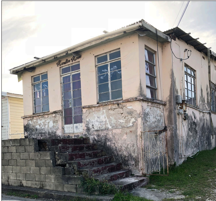
Figure 4: Hamilton House, Bank Hall, Barbados, as seen in 2006, likely built for carpenter Ethelbert O'Connor Scott, who worked on the Panama Canal in the 1910s or 1920s and returned in the 1940s. Scott purchased the property using remittances from Panama. The land was subsequently divided among six family members, some of whom still reside there today. Photograph by Itohan Osayimwese.
