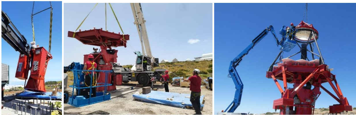
Figure 6. Mounting of the first ASTRI Mini-Array telescope at the Teide observatory. Left: The mounting of the base of the telescope on the foundation. Centre: The mounting of the M1 dish on the azimuth fork. Right: The mounting of M2 support structure (courtesy of EIE Group).
