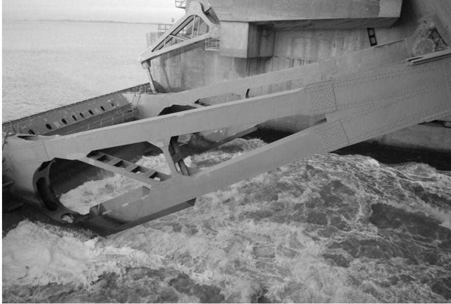
Figure 2.6. One of the 34 gates of the Haringvliet barrier in The Netherlands. This is a tainter valve rotating around a horizontal axis; a hinged support truss (the triangular element visible in the top of the picture) provides the movement, it is driven by a large hydraulic cylinder. Potential vibrations in the same rotation direction can be described by a SDOF system. Picture by Deltares.
