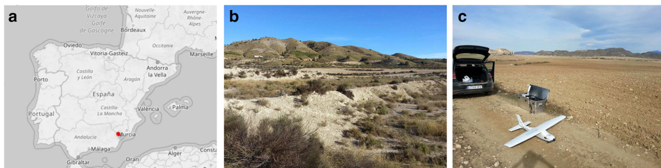
Fig. 1 a The study area is located in the Province of Murcia in southeastern Spain. The photos represent the study area, including the damaged check dams (b), and the UAS (c)
