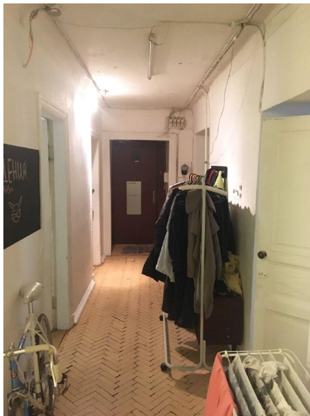
Figure 6. Obshcheye corridor in Agora. The walls have been painted by the tenants. The ceiling lights do not work. Personal belongings (bike, clothes and laundry) are stored outside the rooms.
