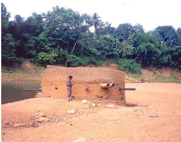
Fig. 5. Impact of sand mining on rural water supply schemes: a water intake structure in Manimala, India, is exposed due to river bed lowering Reprinted from Padmalal et al. (2008).
